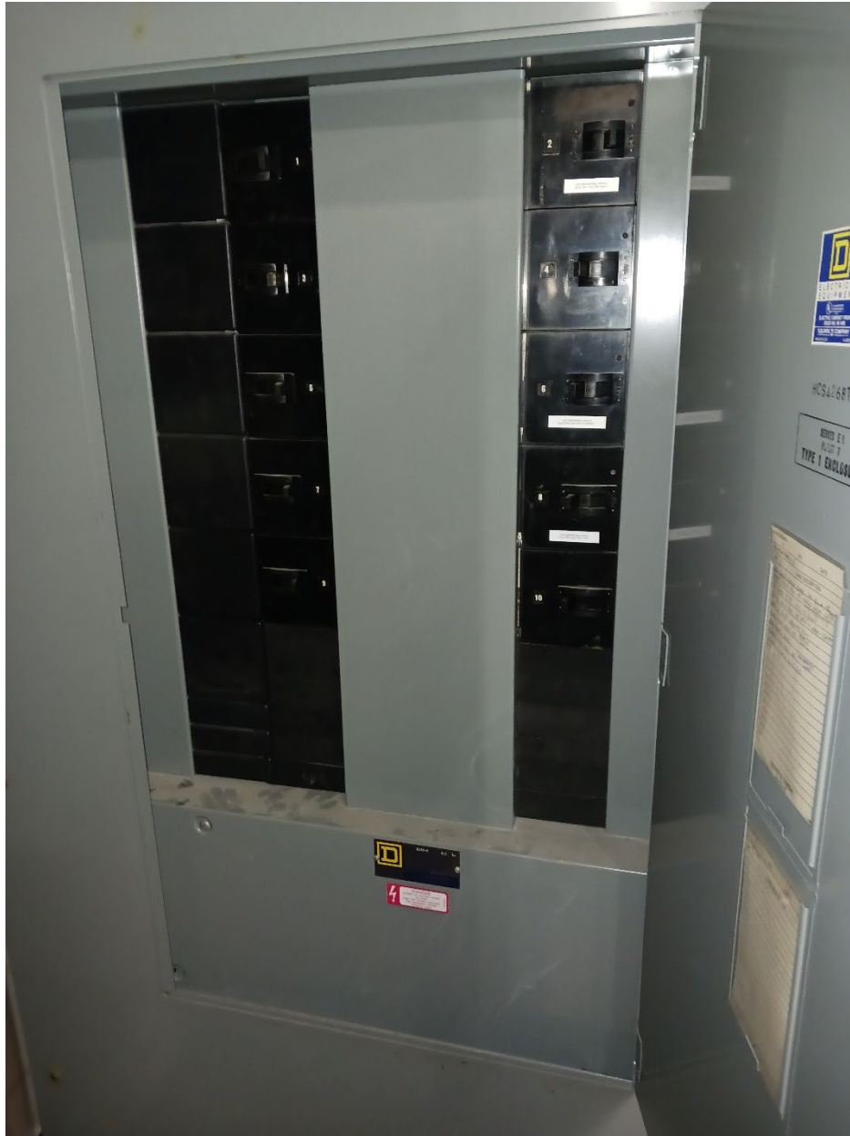
Figure 7: Panel P/A in basement main electrical room E-1
