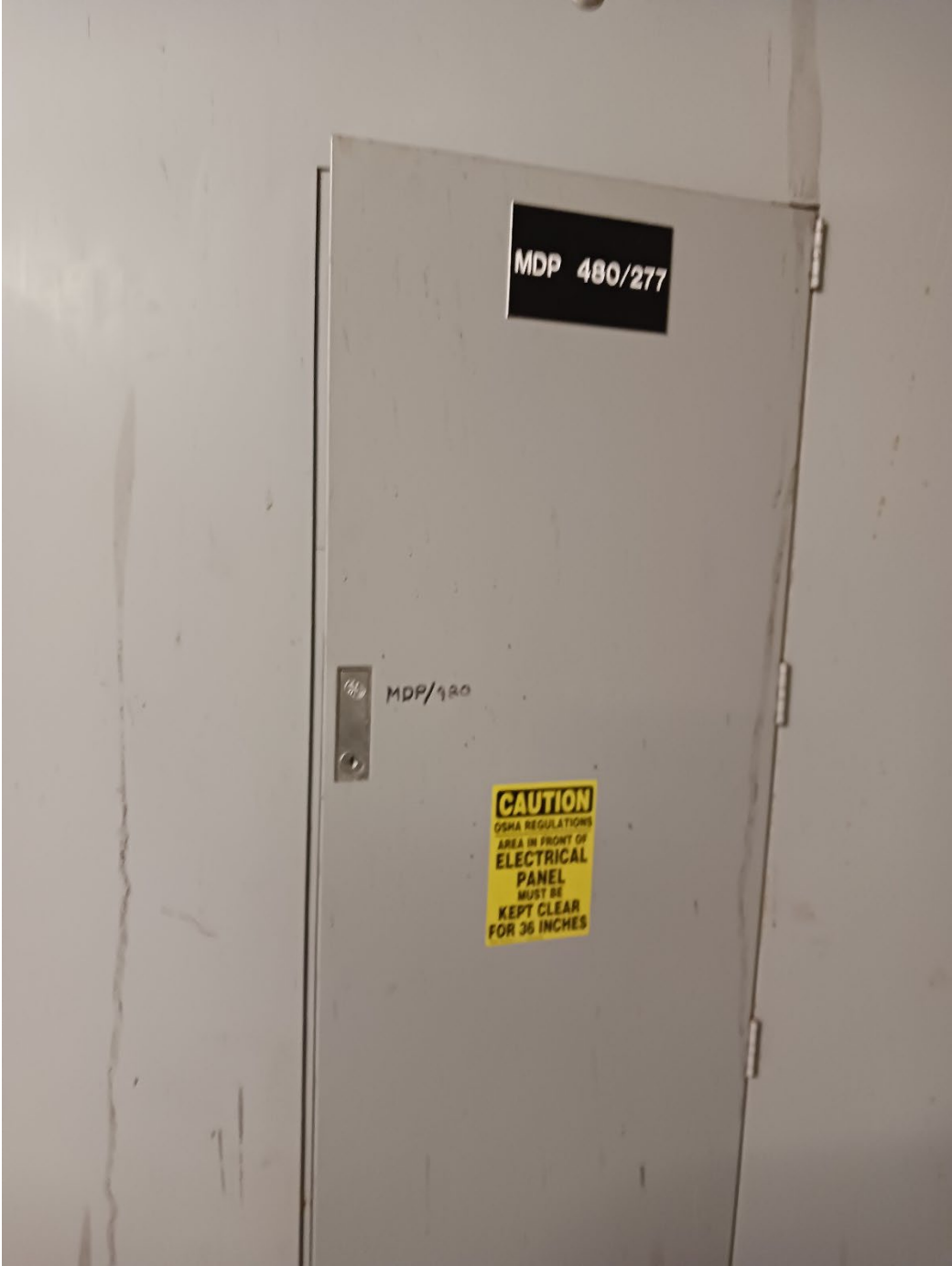
Figure 16: Panel MDP 480 in LEC D Wing basement electrical room
