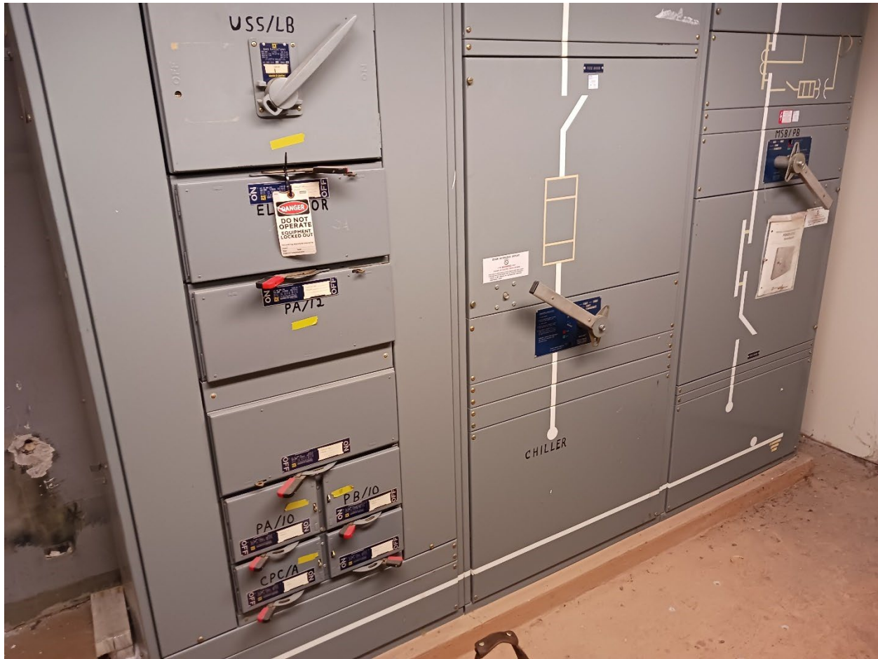
Figure 18: Switchboard MSB/PB in Twelfth Floor Electrical Room
