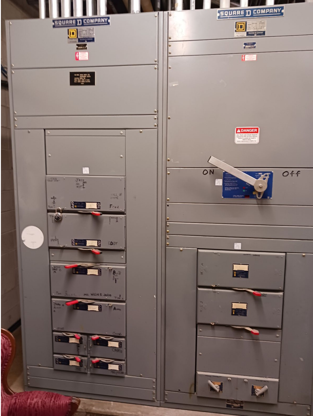
Figure 4: Left side of Switchboard PMB in basement main electrical room E-1
