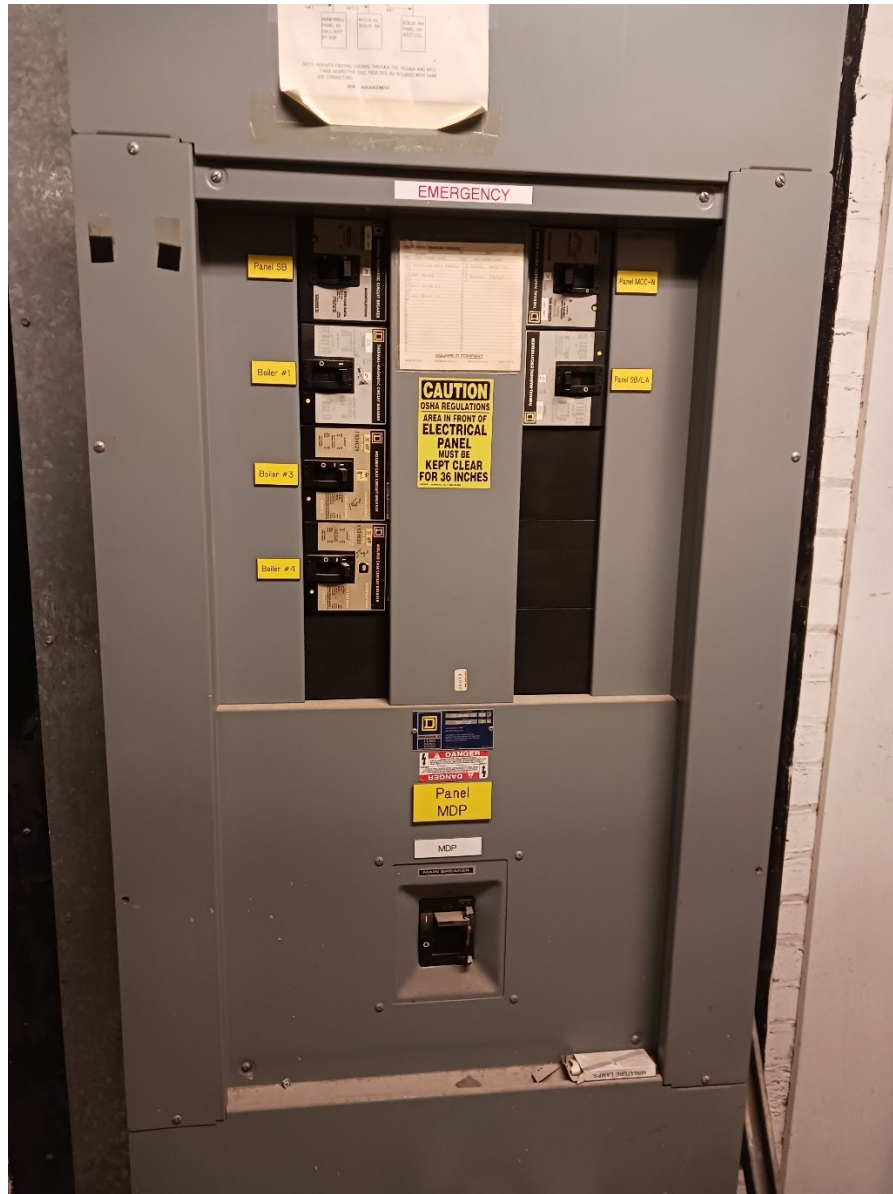
Figure 2: Panelboard MDP in Courthouse basement boiler room
