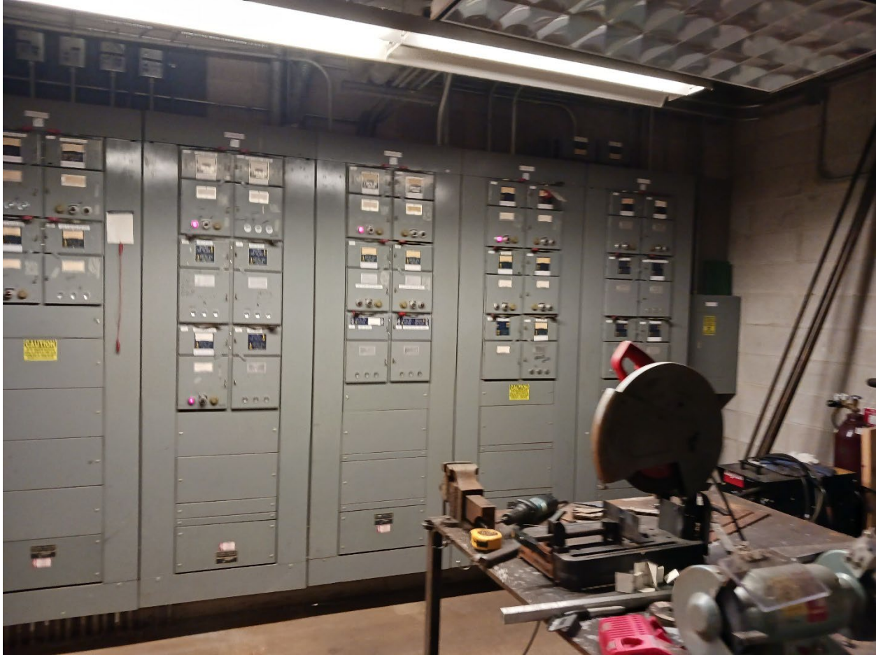
Figure 9: Motor Control Center MCA-E in basement boiler room
