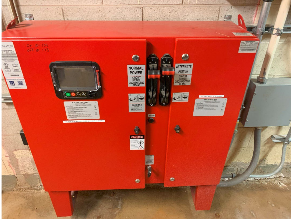
Figure 9: Courthouse Fire Pump Controller in subbasement fire protection room
