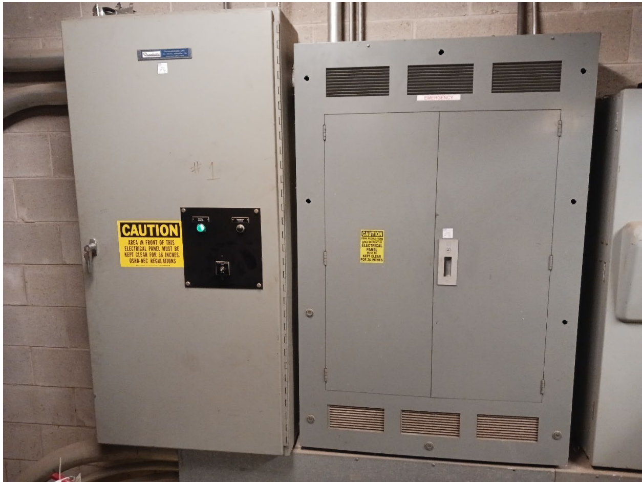
Figure 7: ATS #1, Panel EP/B in basement generator room
