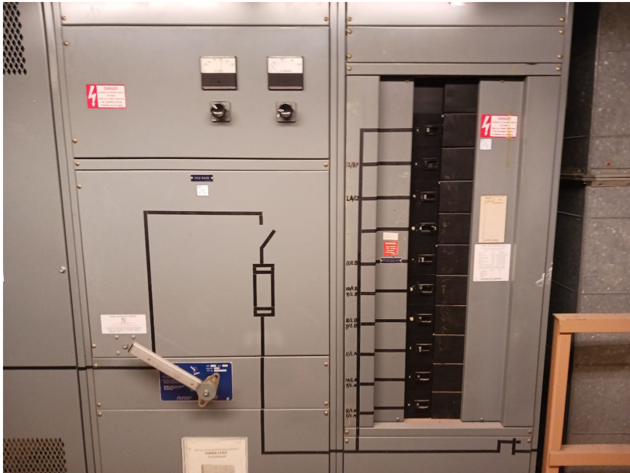
Figure 19: Unit Substation USS LB in Twelfth Floor Electrical Room
