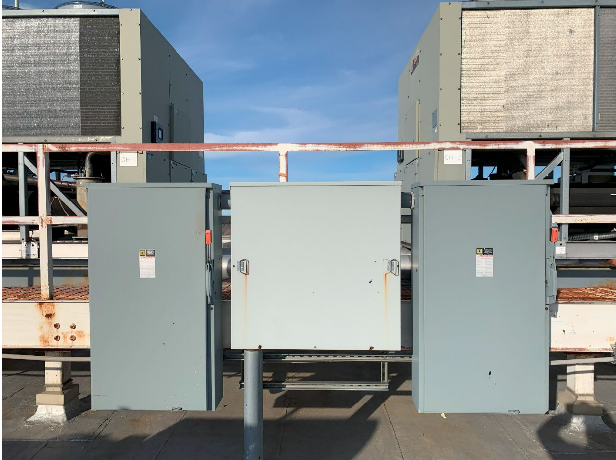
Figure 24: Courthouse Roof Top Chiller CH-1 and CH-2 Disconnects
