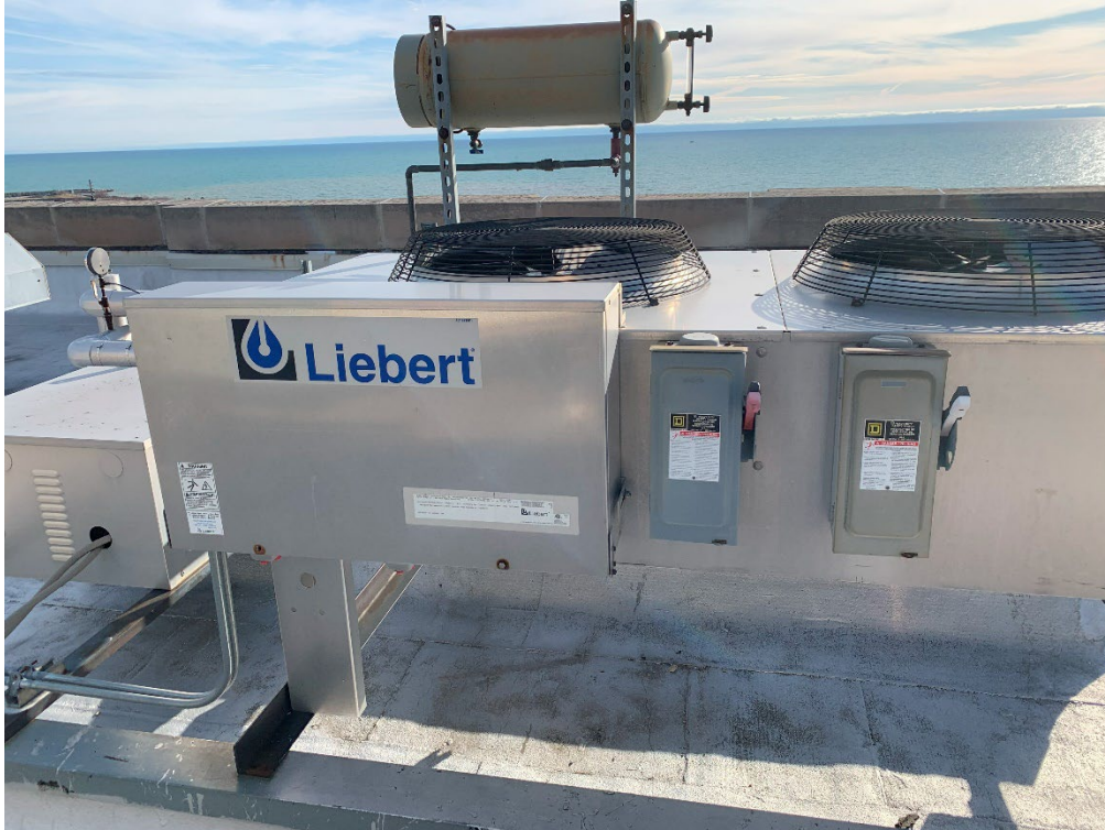
Figure 26: Courthouse Roof Top Liebert Unit
