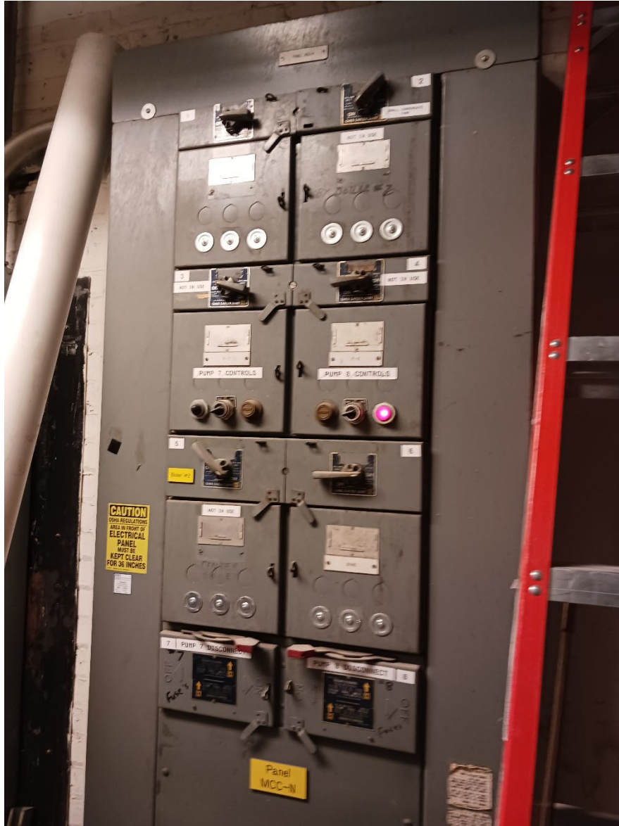
Figure 3: Motor Control Center MCC-N in Courthouse basement boiler room
