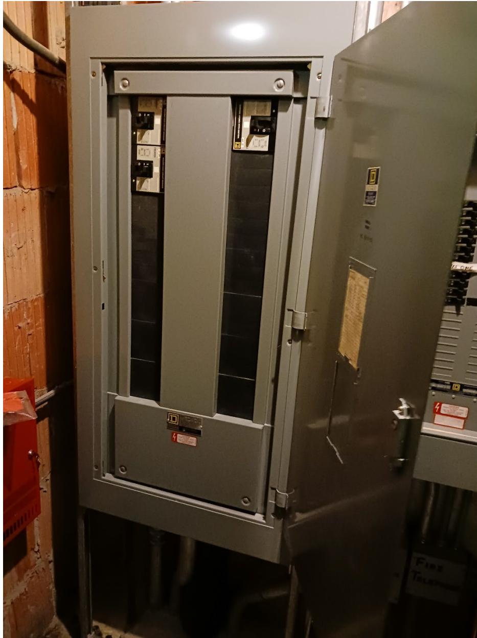
Figure 14: Panelboard 5/PA in fifth floor electrical closet
