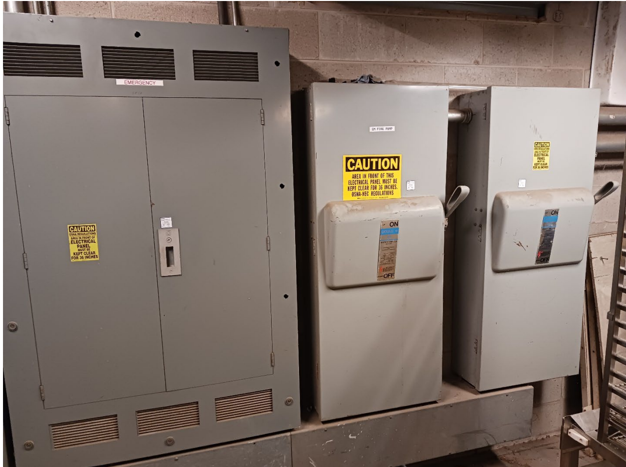
Figure 8: Panel EP/B, 600A Fire Pump Disconnect, 600A Panel EP/B disconnect
