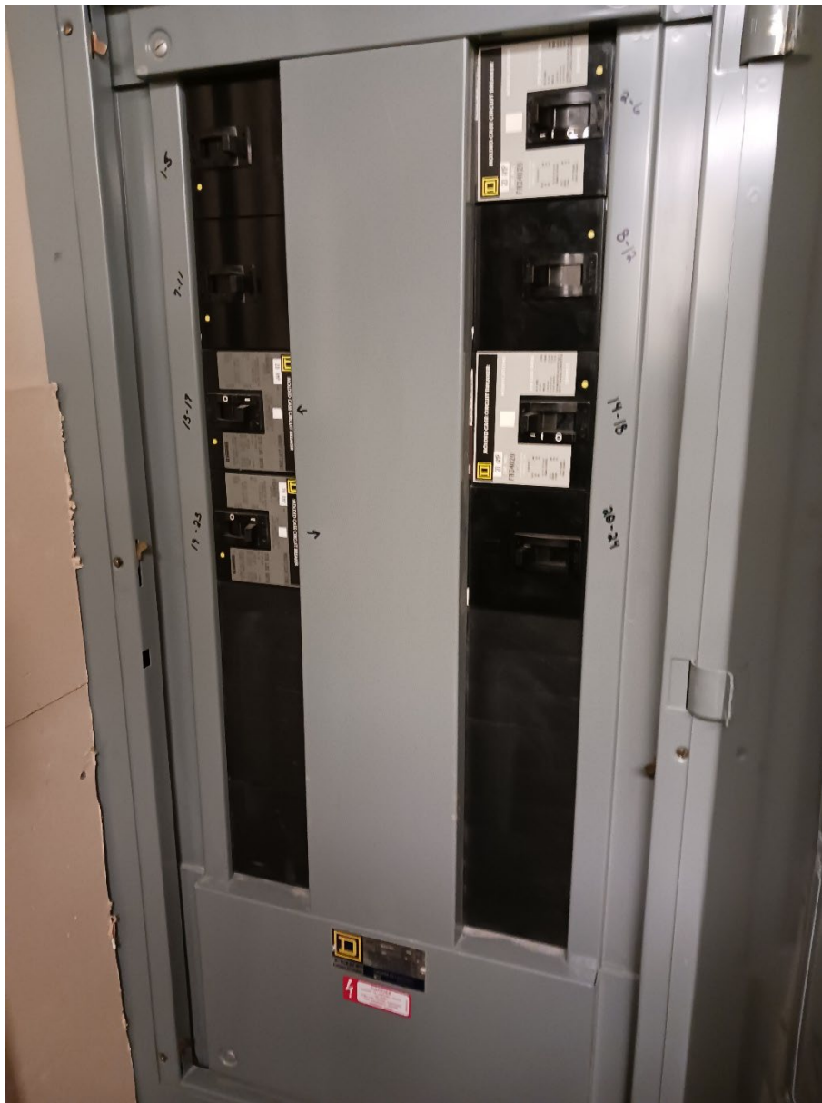
Figure 12: Panelboard 2/PA in first floor electrical closet
