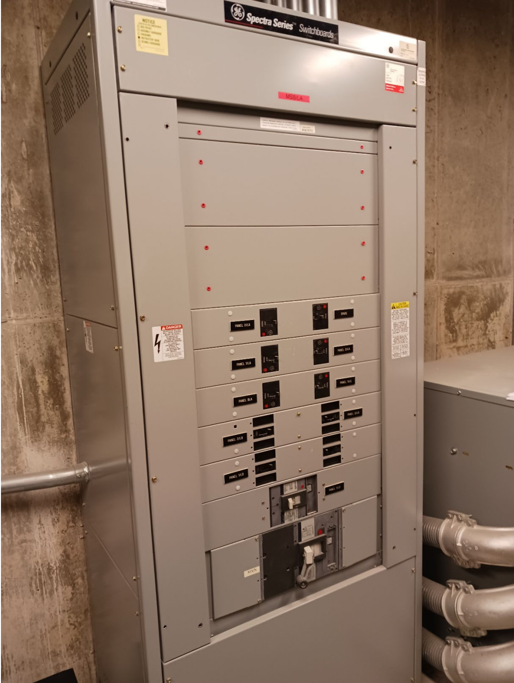
Figure 19: 1200 Amp MSB/LA in LEC D Wing basement LE06 electrical room
