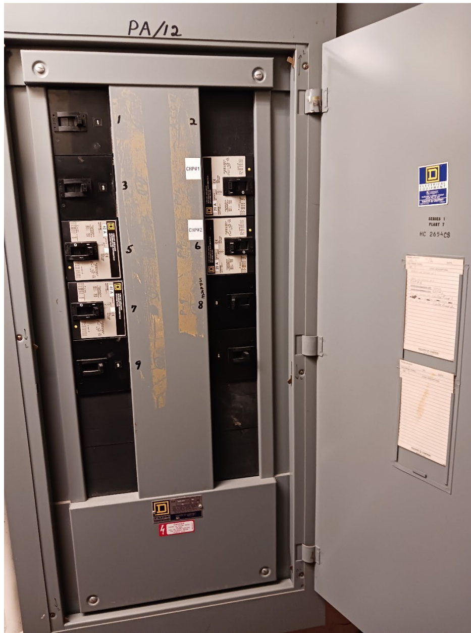
Figure 21: Panel 12/PA in Twelfth Floor Electrical Room
