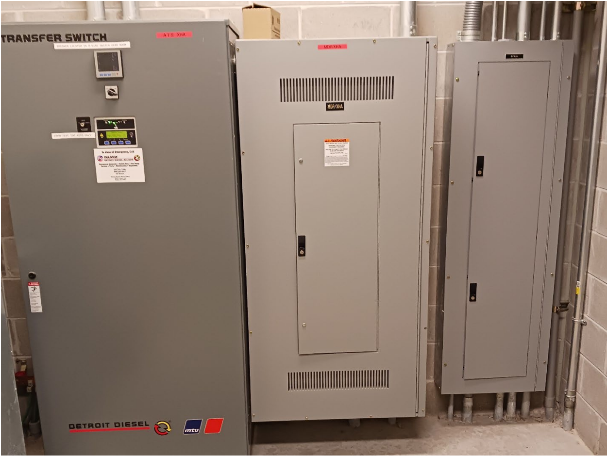
Figure 20: ATS XHA, MDP/XHA, B/ELA in LEC D Wing basement LE07 electrical room
