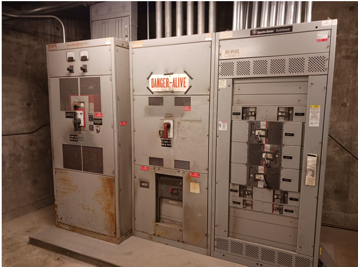
Figure 14: Switchboard MSB B in LEC D Wing basement electrical room
