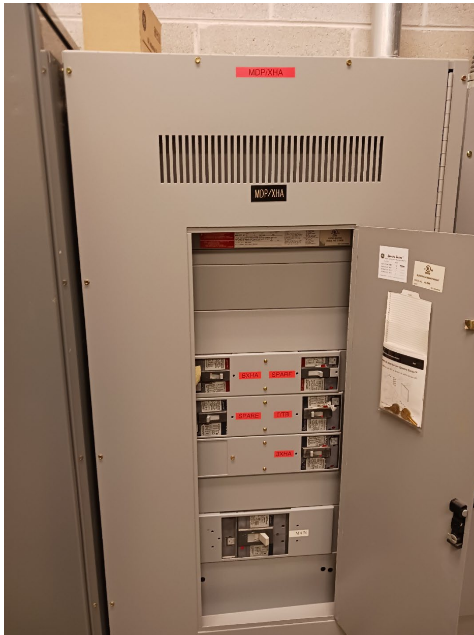
Figure 21: Panel MDP/XHA in LEC D Wing basement LE07 electrical room
