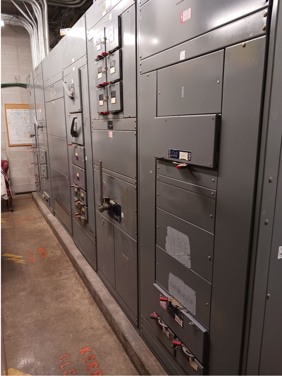
Figure 3: Switchboard PMB in basement main electrical room E-1
