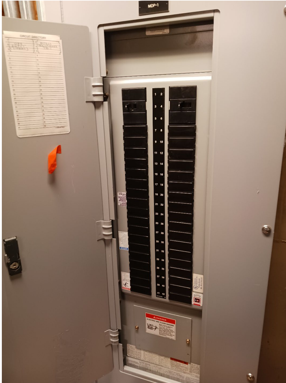
Figure 22: MDP-1 Distribution (Cutler-Hammer PRL2A, 277/480Y, 225A)
