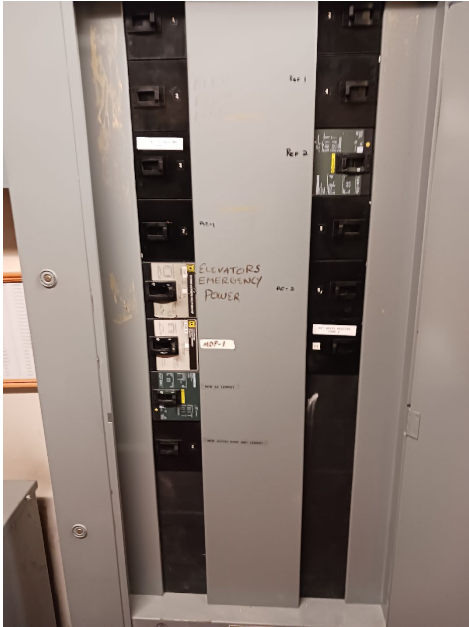
Figure 20: Panel 12/EP in Twelfth Floor Electrical Room
