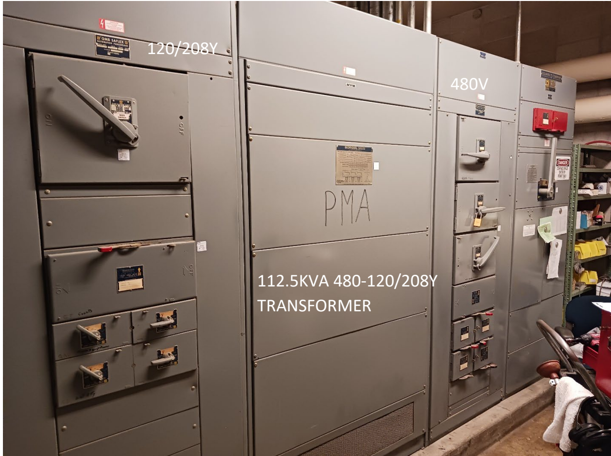
Figure 2: Switchboard PMA in basement electrical room
