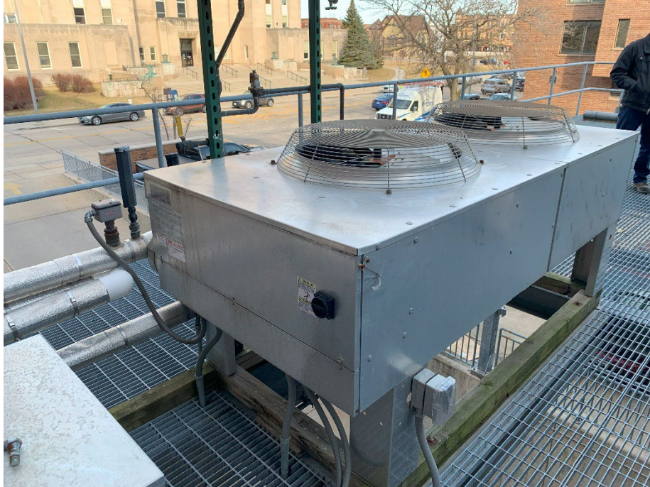
Figure 23: LEC Liebert Unit on Chiller Platform
