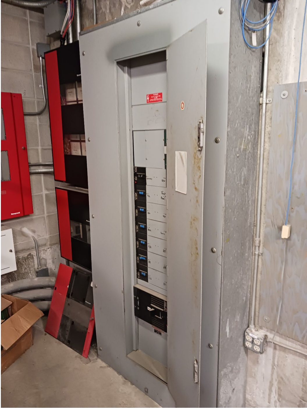
Figure 18: Panel MDP 208 in LEC D Wing basement electrical room
