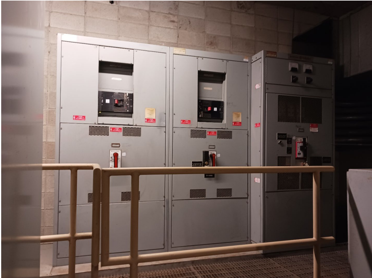
Figure 1: Switchboard MSB A (left side) in basement electrical room
