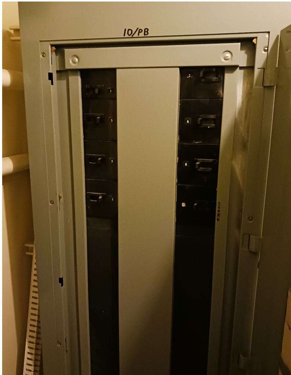
Figure 17: Panelboard 10/PB in tenth floor electrical closet
