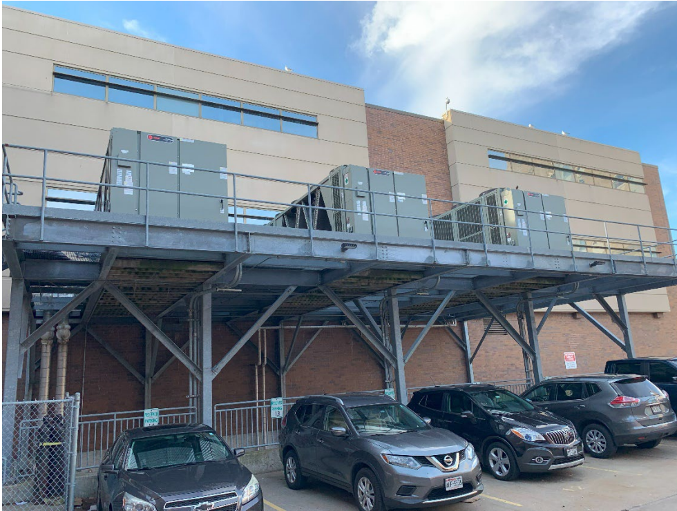
Figure 22: LEC Chiller Platform for Chiller CH-1, CH-2 and CH-3
