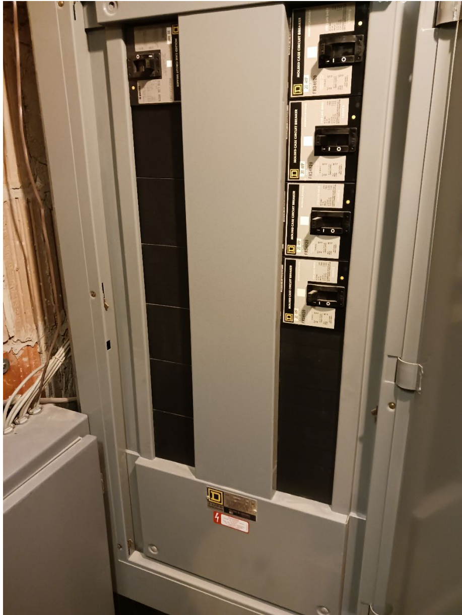
Figure 13: Panelboard 2/PB in second floor electrical closet
