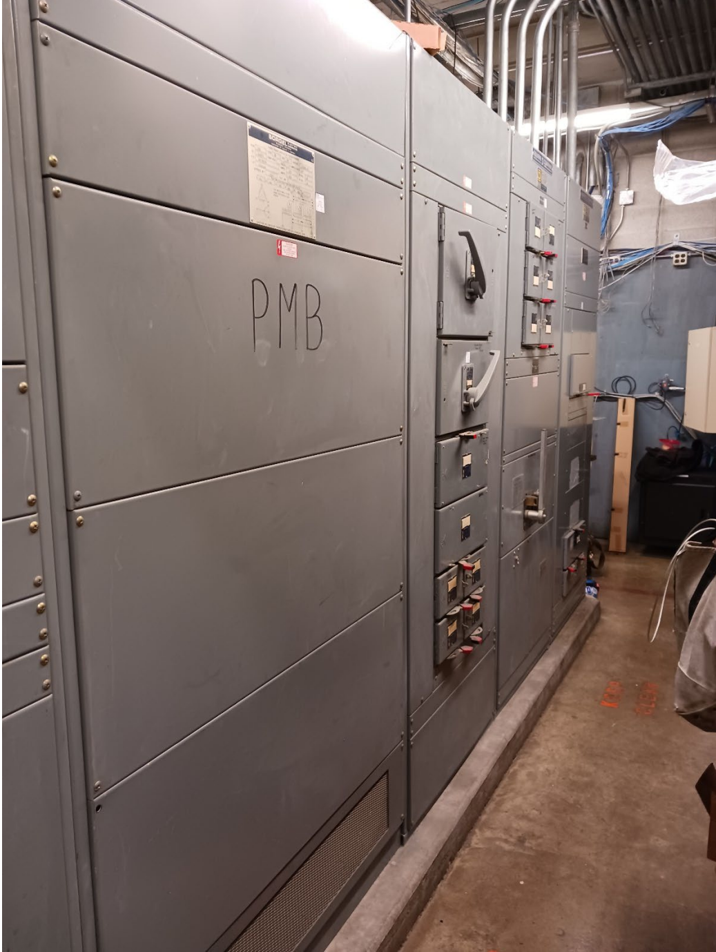
Figure 5: Right side of Switchboard PMB in basement main electrical room E-1
