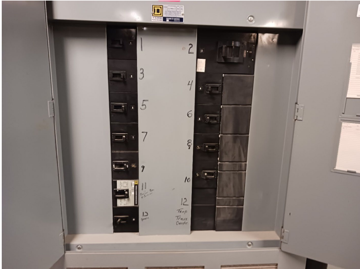
Figure 10: Panelboard EP/B in basement generator room
