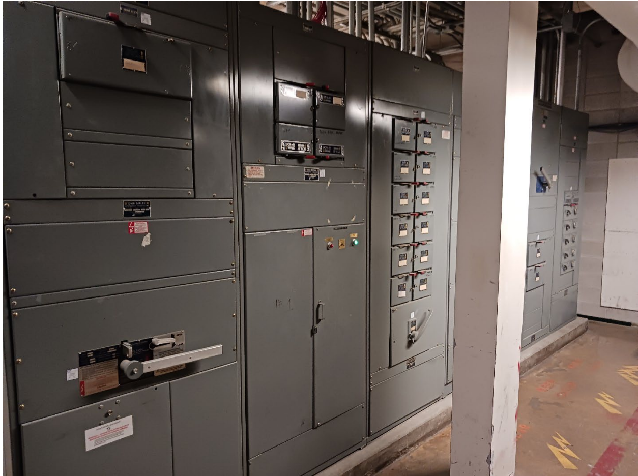
Figure 6: Switchboard PME in basement main electrical room E-1
