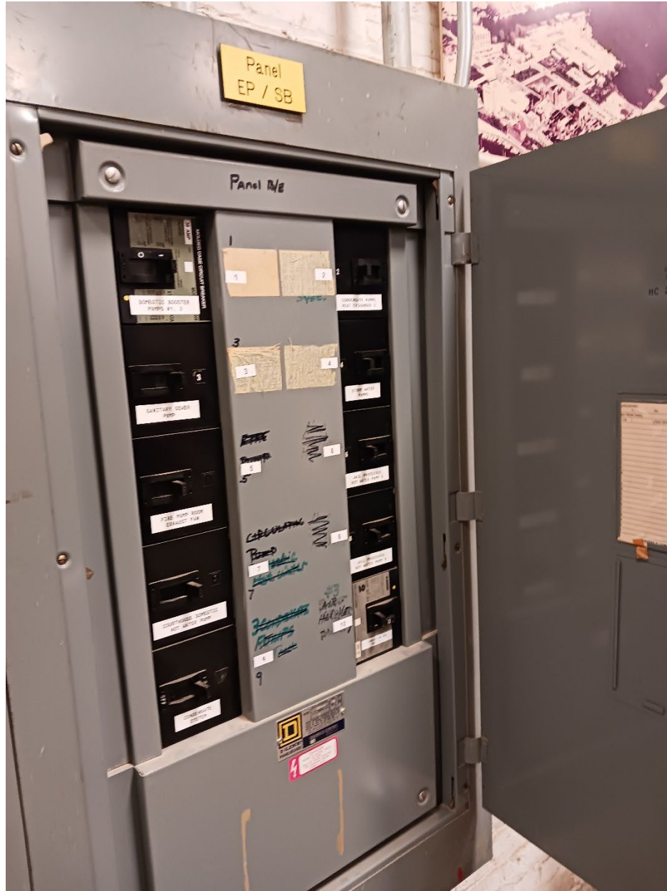
Figure 4: Panelboard EP/B in subbasement maintenance shop
