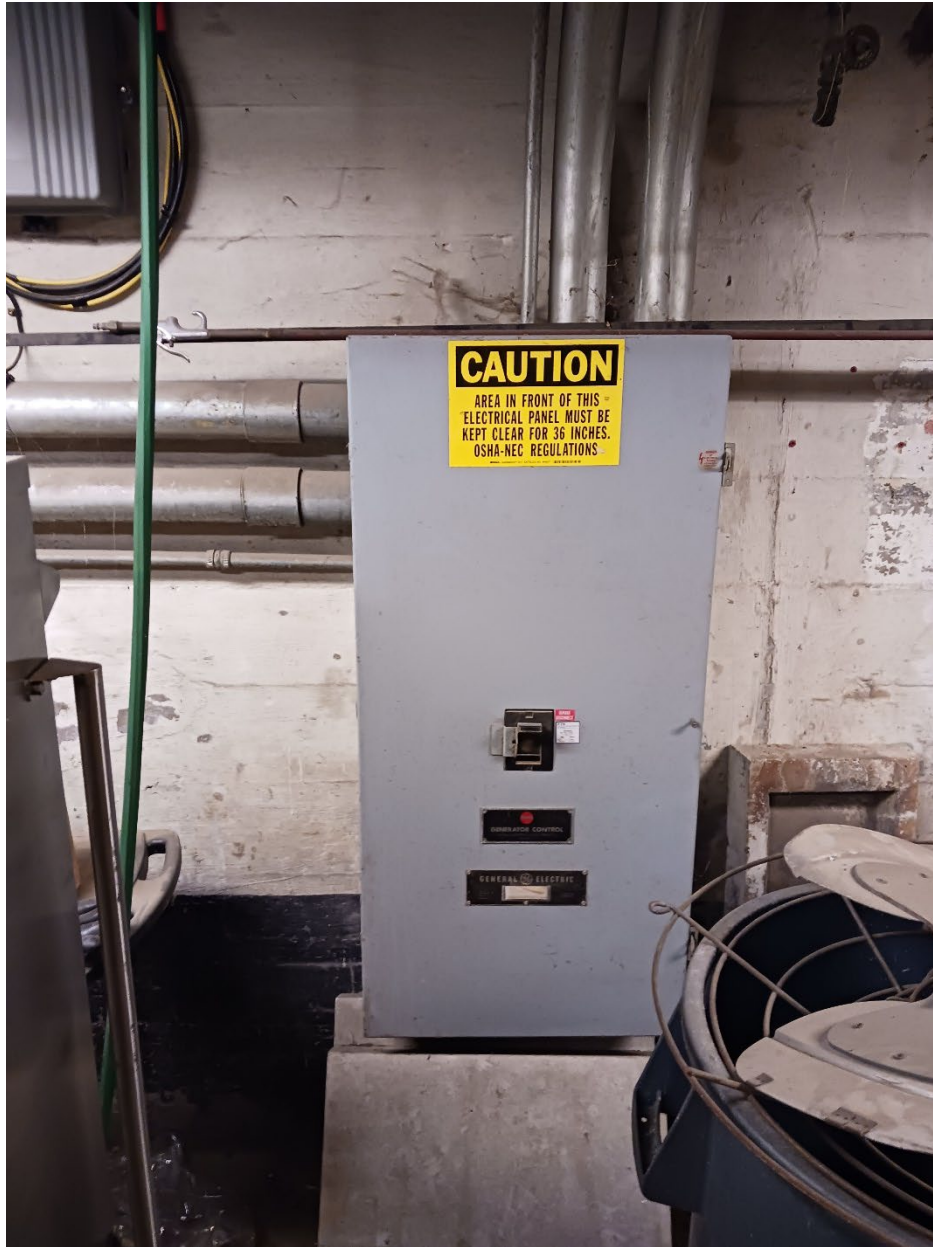
Figure 6: Generator 700A circuit breaker (GE) in basement generator room
