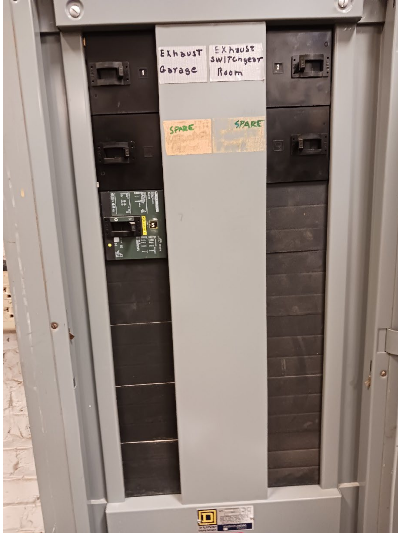
Figure 5: Panelboard SB/PA in subbasement maintenance shop
