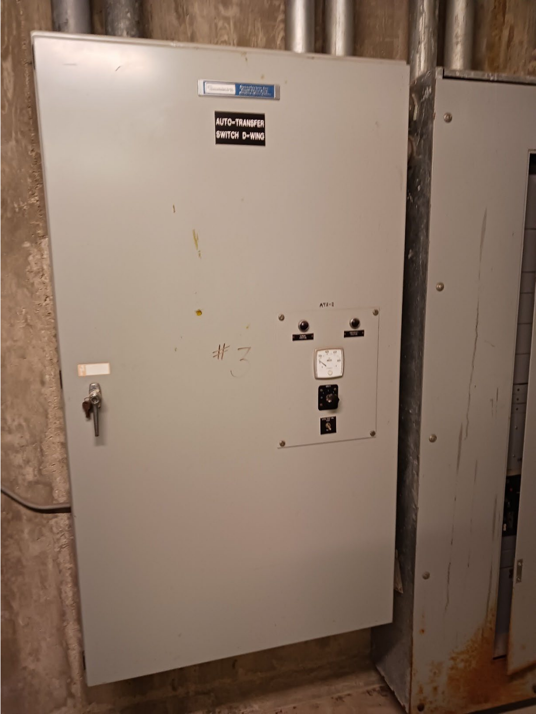
Figure 15: 800 Amp ATS in LEC D Wing basement electrical room
