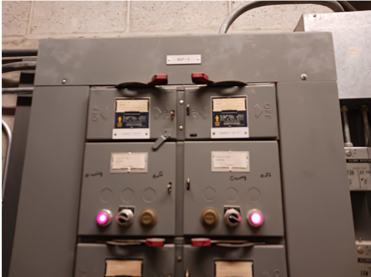
Figure 13: Panel MCP-E in mechanical penthouse
