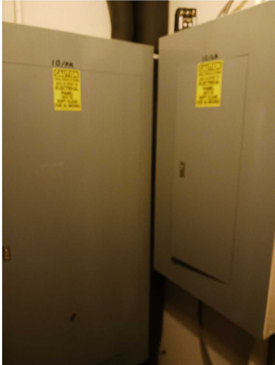
Figure 16: Panelboard 10/PA in tenth floor electrical closet
