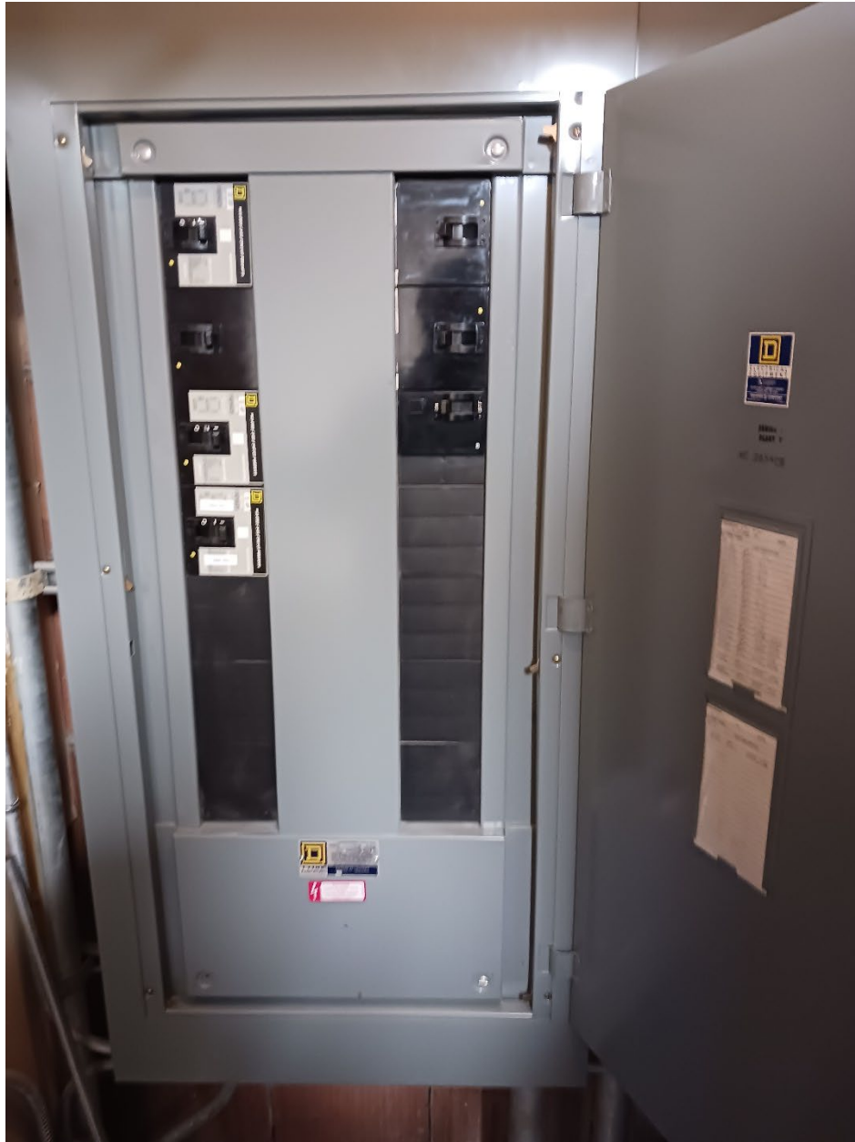
Figure 15: Panelboard 5/PB in fifth floor electrical closet
