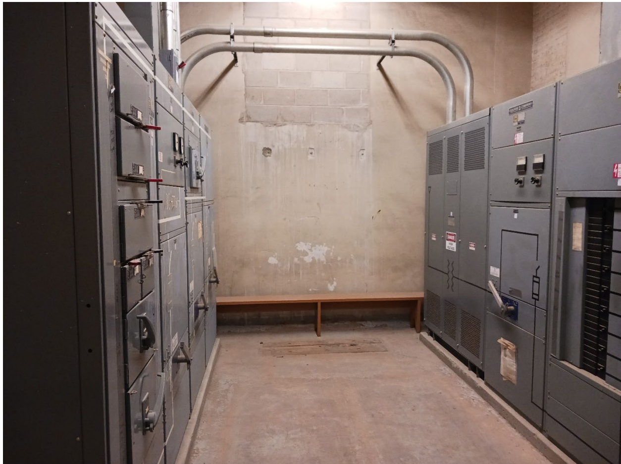
Figure 1: Switchboard MSB/PA on left, USS LA on right in subbasement electrical room
