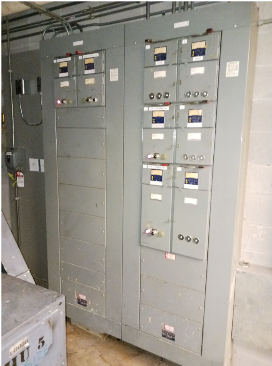
Figure 11: Motor Control Center MCB-N in Kitchen mechanical room
