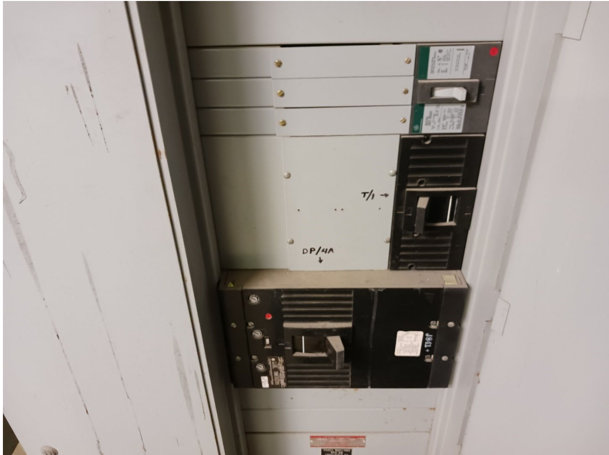
Figure 17: Panel MDP 480 in LEC D Wing basement electrical room
