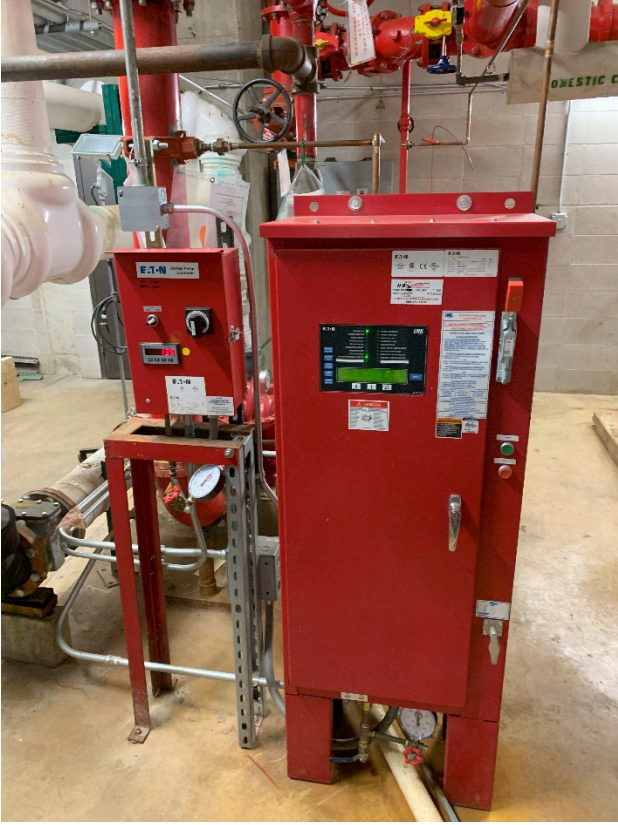
Figure 10: LEC Fire Pump Controller in basement
