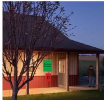
Disconnect 2 located on exterior of home.
