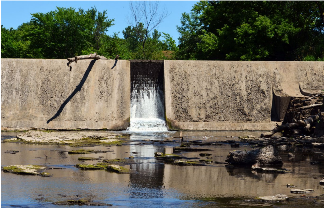
Figure 34: Horlick Dam exposed stoplogs during extreme low flow in 2012 (photo credit: Erick Walquist)
