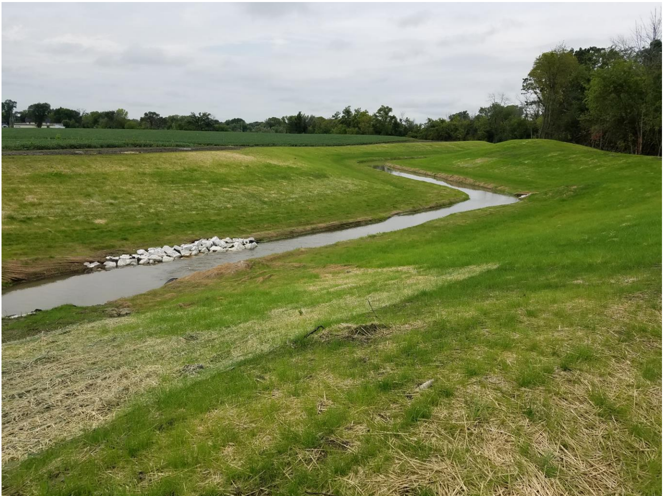
Oakcrest Creek Restoration – Remove legacy sediment, grade/seed eroding banks, create two-stage channel
