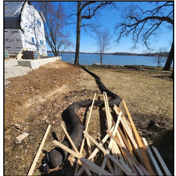
INCORRECTLY INSTALLED SILT FENCE.
