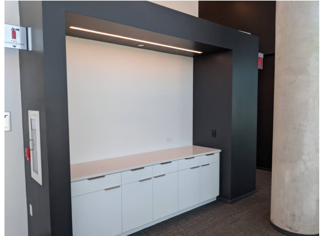
Complete tile and countertop installation in pantry and lobby areas throughout building
