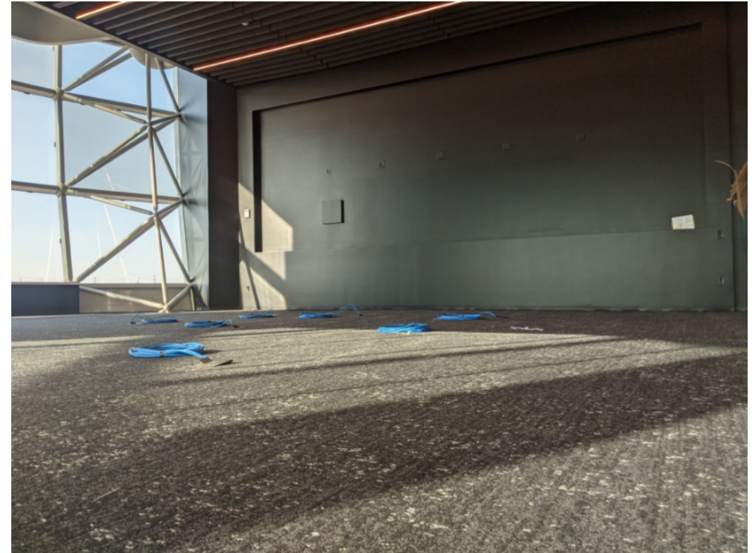
Complete drywall, painting and flooring installation in Network Operation Center (NOC) on Level 2
