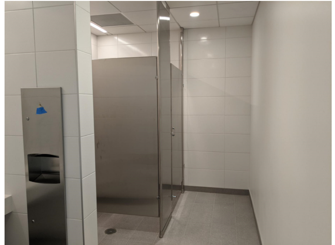
Complete installation of toilet partitions and accessories in restrooms throughout the building
