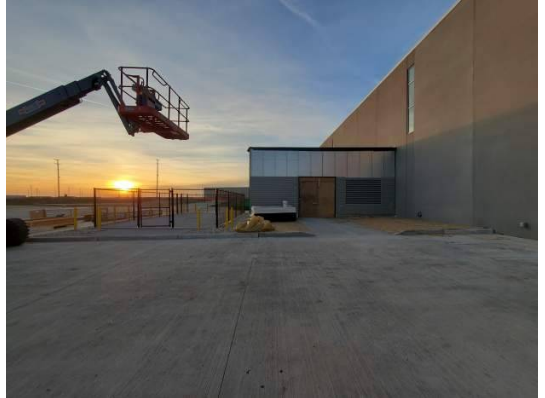
Exterior Bump-out and Bulk Tank Pads
