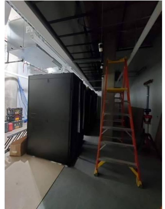
Server Rack Installation in Lower-Level Telecommunications Room
