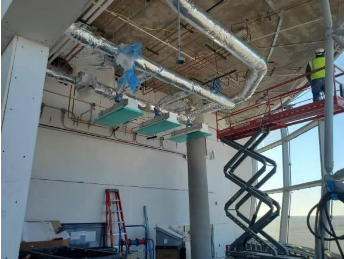
Board Room Overhead MEP Installation
