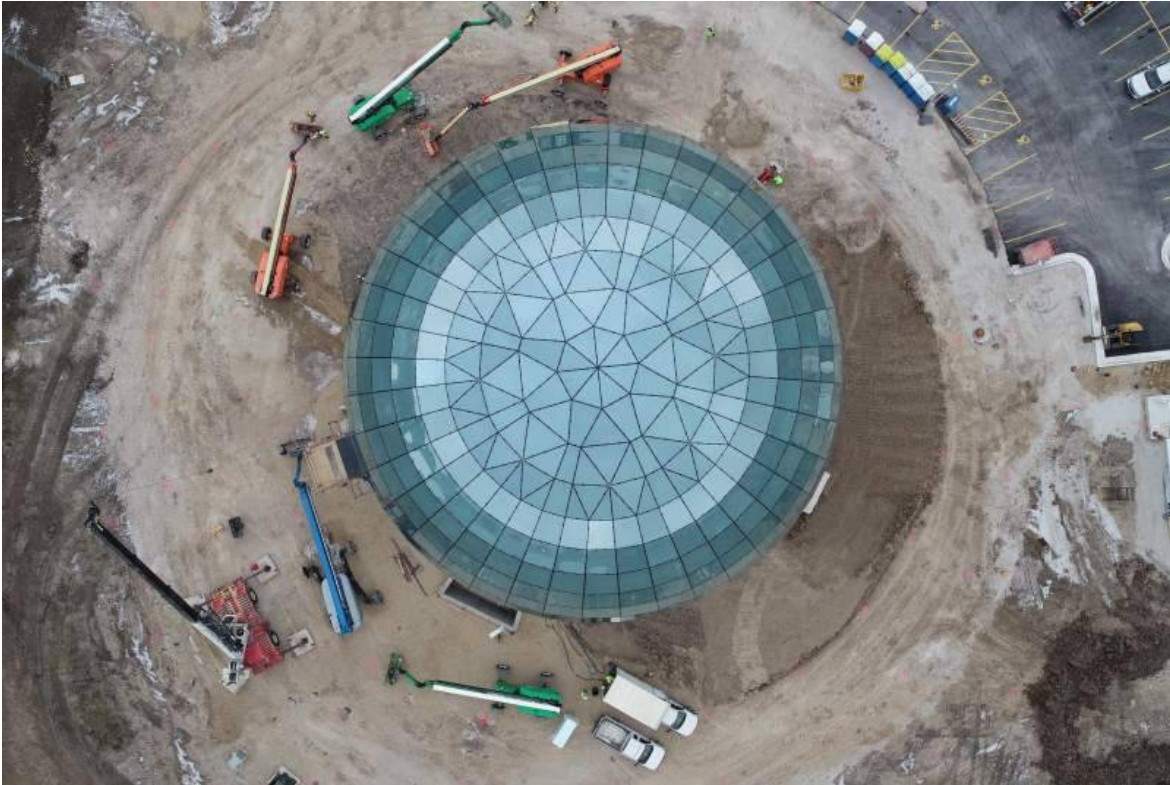
Aerial View of the HPC DC
