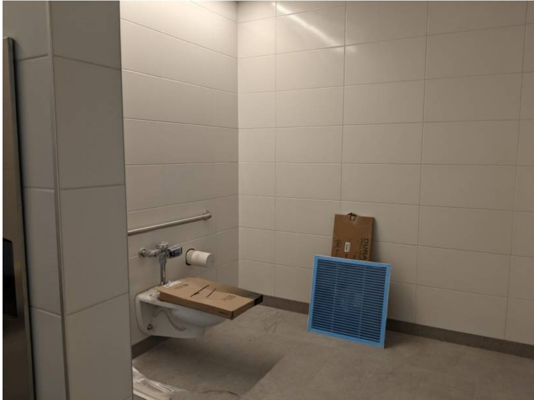
Complete tile installation and begin installation of toilet specialties in Level 2 restrooms
