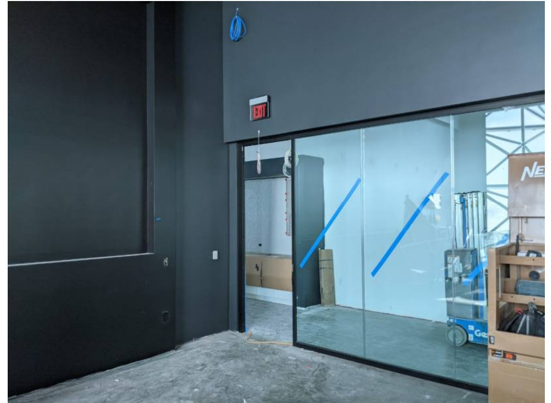
Complete paint and glass installation in Network Operation Center (NOC) on Level 2
