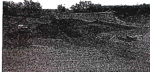
Foundry sand being incorporated as part of grading activities during reclamation of the Foley Pit (Photo by Dave Misterek, DNR)
