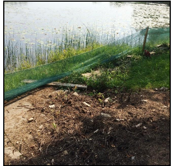
INCORRECTLY INSTALLED SILT FENCE.
