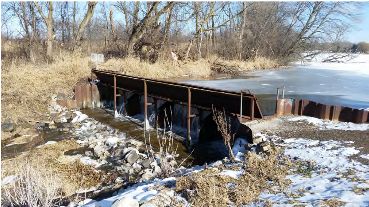
Dam located on the west side of Eagle Lake has a spillway elevation at 795.57 feet.
