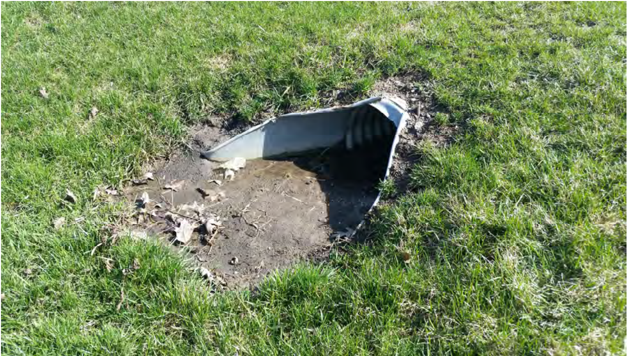
Sediment in culvert that leads to Eagle Creek on Hwy 75
