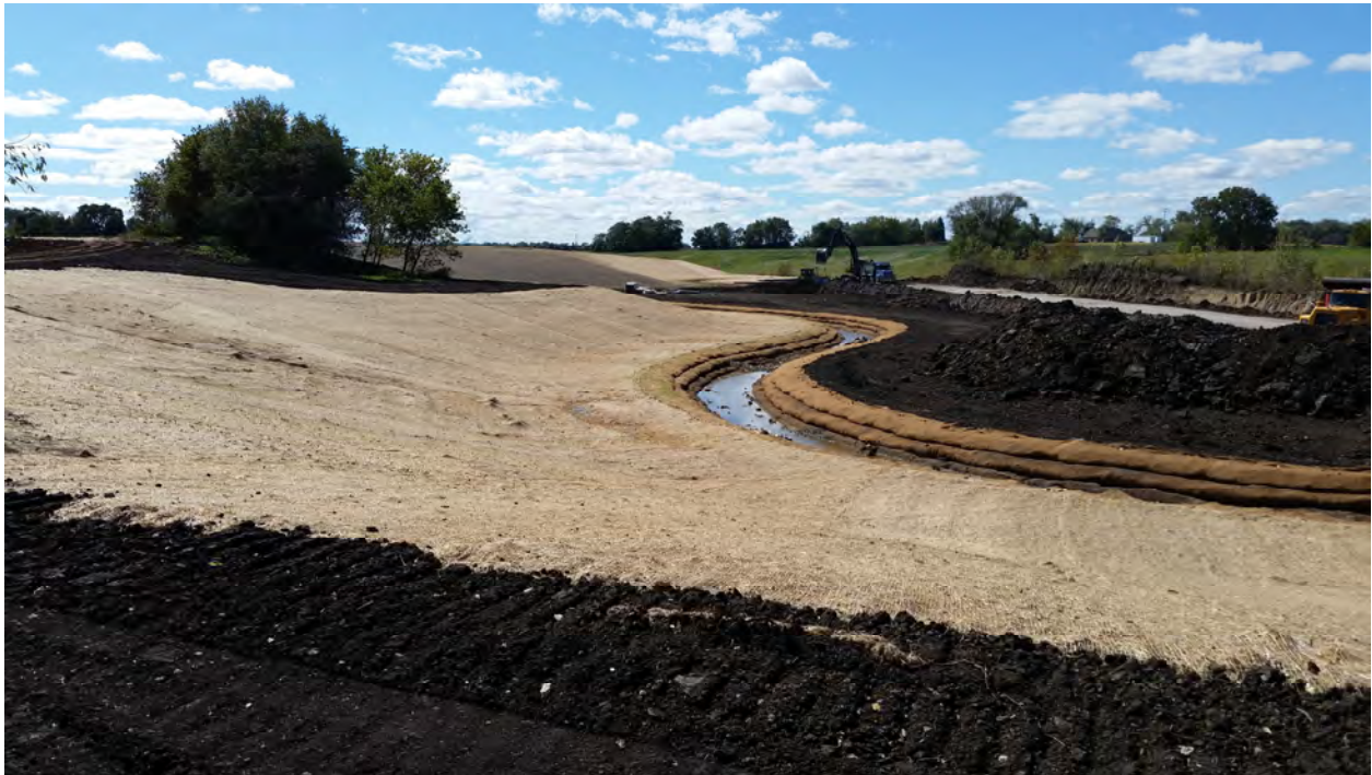
During construction of a 2 stage channel on the Pike River in Racine County (above)
