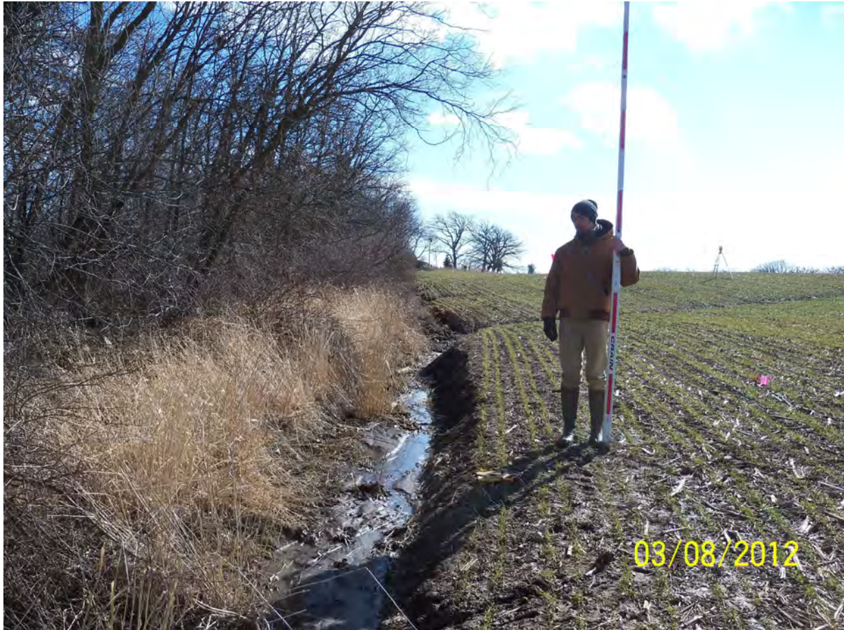
GULLY EROSION IN FIELD #2403
