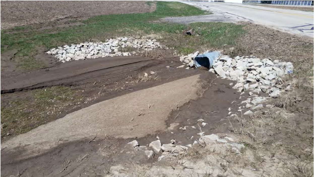
Sediment from cropland in catch basin and culvert – needs to be cleaned out
