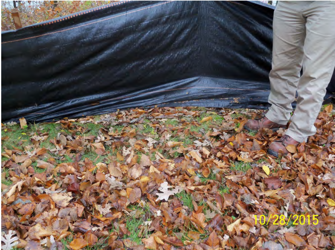
Silt fence improperly installed on Eagle Lake construction, not trenched into ground
